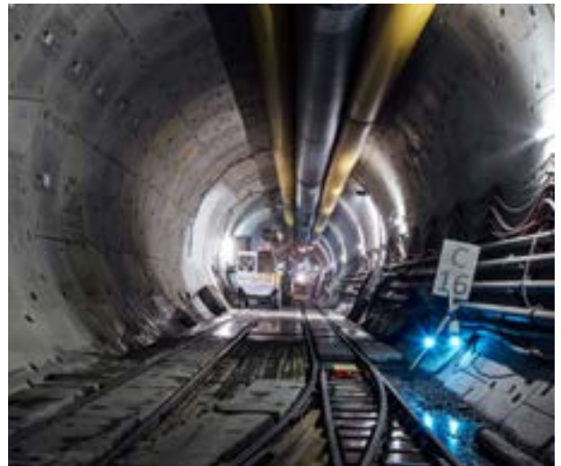
The Koralm Tunnel will be the sixth longest railway tunnel in the world.
